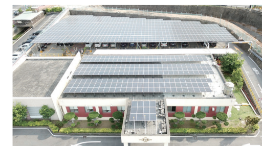
Solar power generation equipment, Taiwan Copper Foil Co., Ltd.
