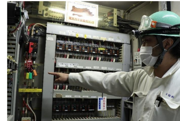
Operation and review of the lockout system
