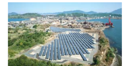
Solar power plant, Hikoshima Smelting Co., Ltd.
