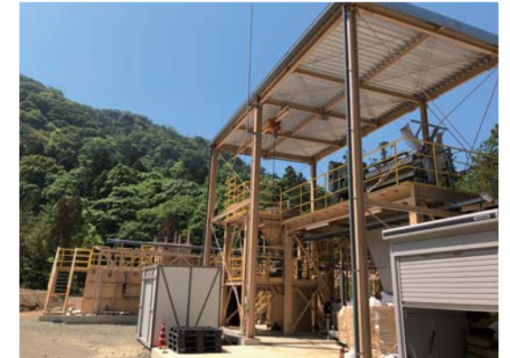
New acidic water treatment equipment has started operations. (Udo Mine)
